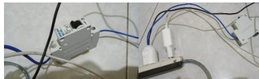
FIGURE 11. Circuit connected with MCB
